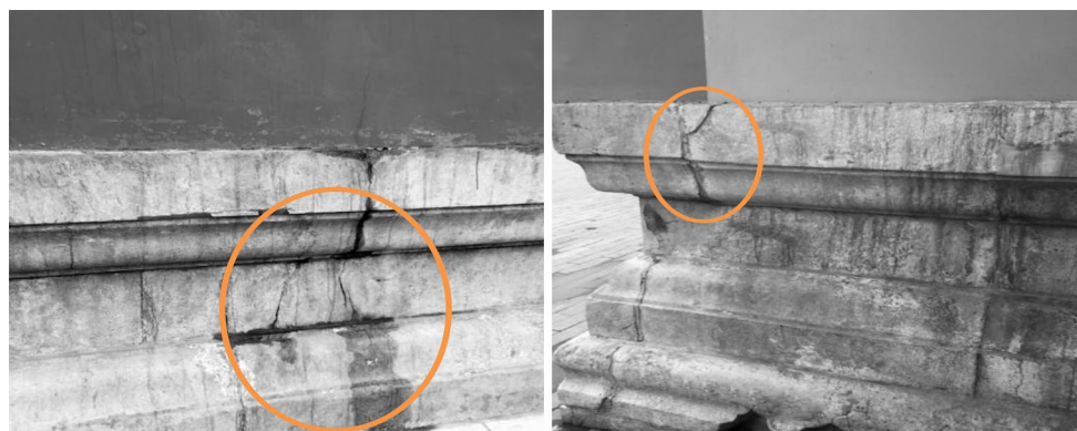
Fig. 3 Seepage and cracks at the foot of the wall
