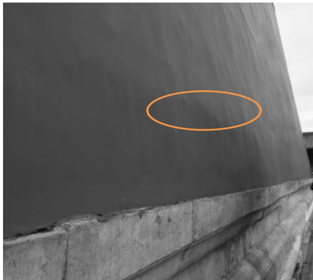
Fig. 9 Local bulging of ancient wall
